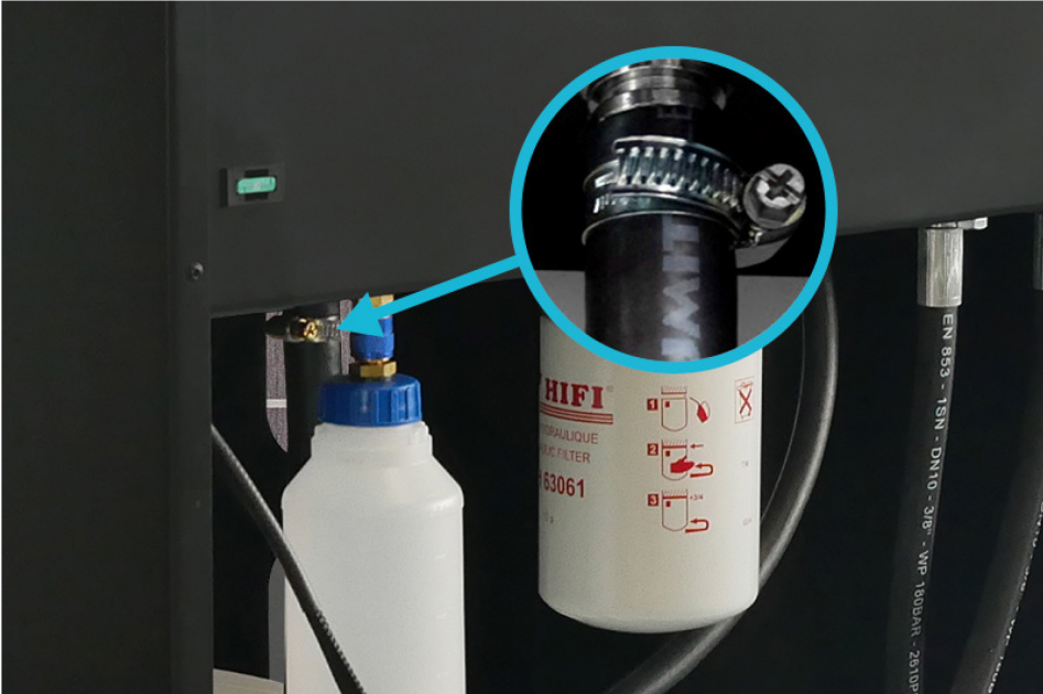
Figure 25. A clamp used to adjust the length of the suction line.
